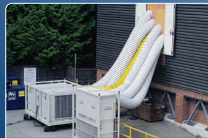
Telco Hub Cooling
