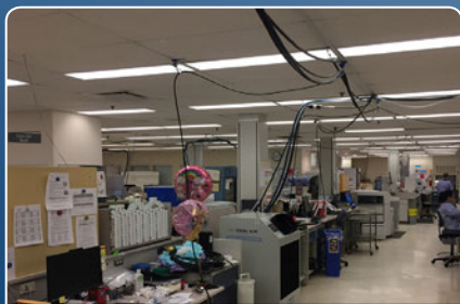
Large Scale Lab Cooling
